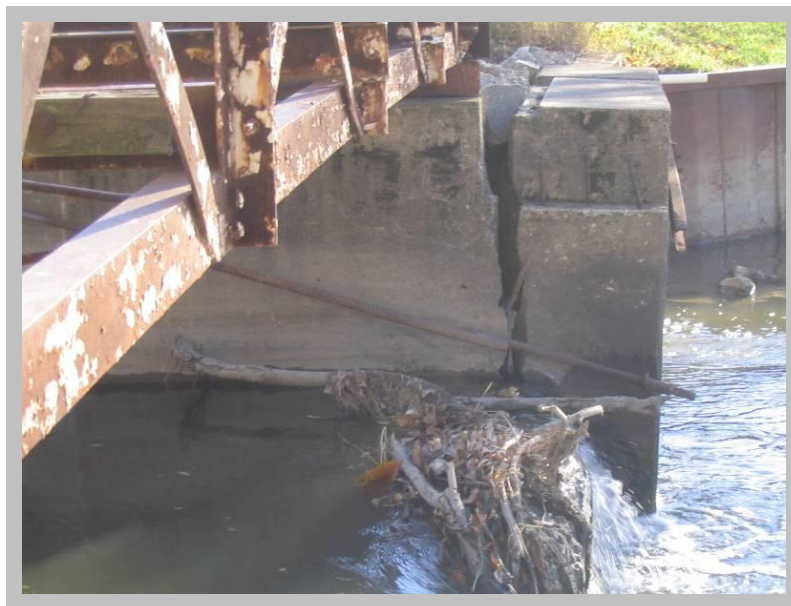
Figure 2- 3 - Left abutment, significant crack
