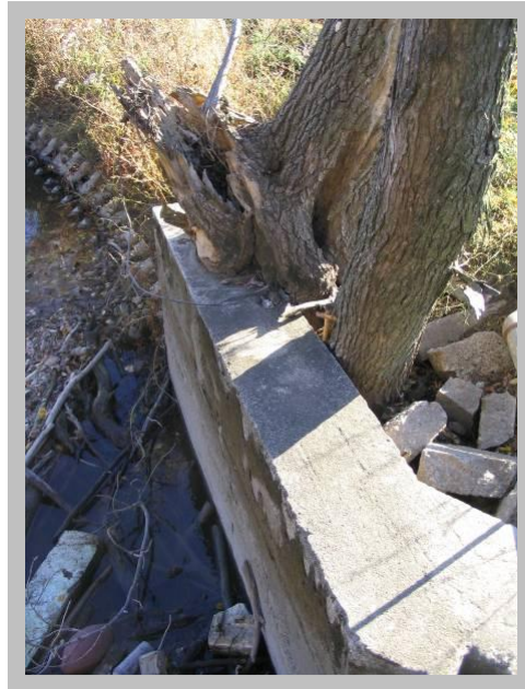
Figure 2-4 - Mature Tree compromising left training wall
