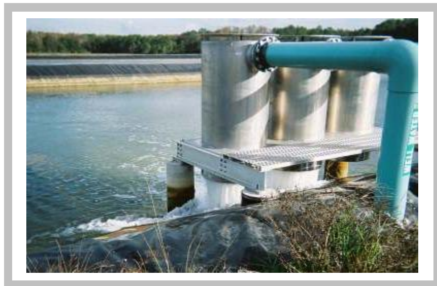
Figure 5-1 - Mechanical Aeration Display
