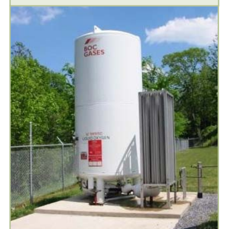
Typical liquid oxygen tanks
