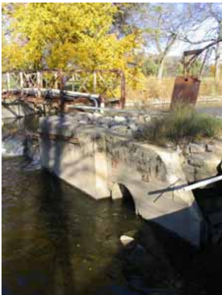
Figure 2.3: View of left abutment and culvert, the steel gate can be seen in the upper right
