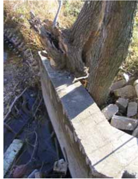
Figure 2.2: Mature tree compromising left training wall
