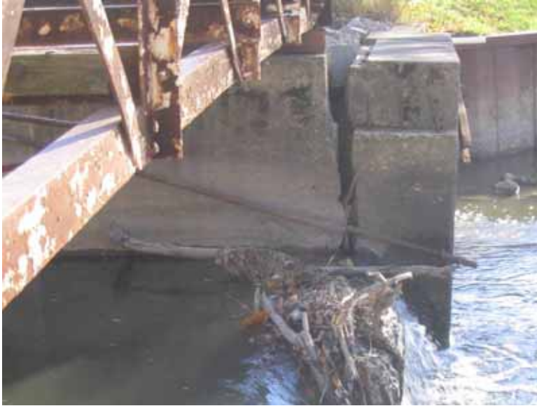
Figure 2.1: Left abutment, significant crack
