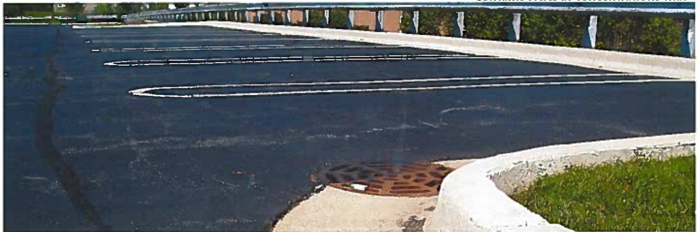
Figure 1: Sealcoat is the black liquid sprayed onto the asphalt pavement of some parking lots, driveways, and playgrounds. The sealcoat product predominantly used in the central, southern, and eastern U.S. contains coal tar, a known human carcinogen.
